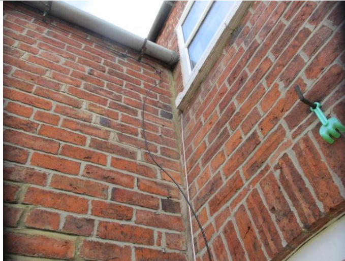
Structural cracking to rear return.
