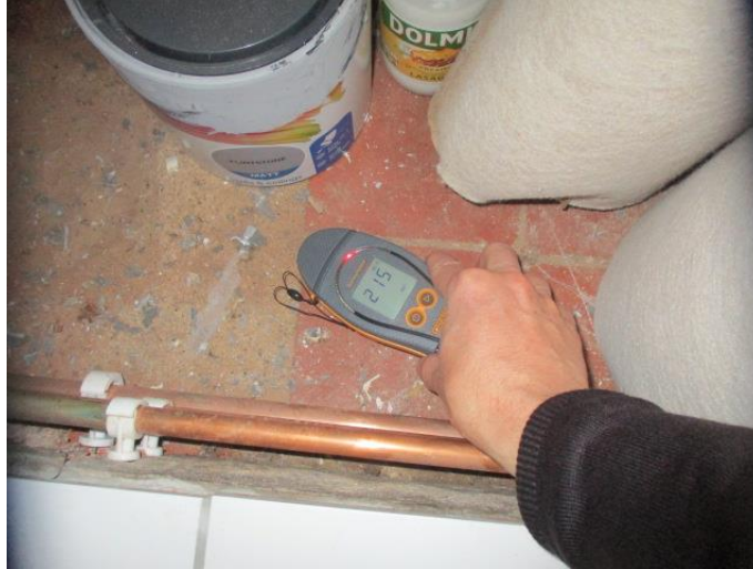
Damp to the floor in the under stairs cupboard.
