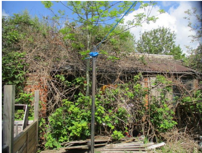
Overgrown and dilapidated outbuildings.
