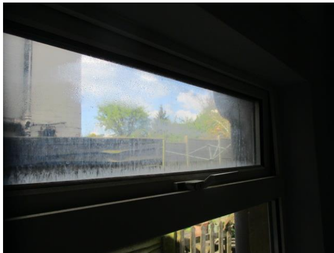
Failed window unit.
