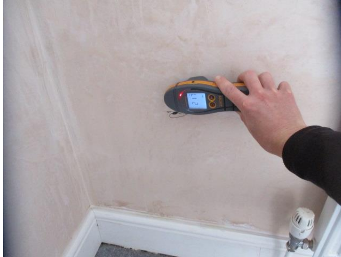
Damp to newly plastered wall.
