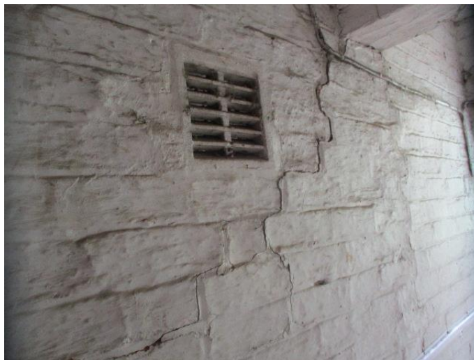
Structural cracking to passageway.
