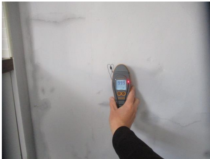
Damp to kitchen wall.
