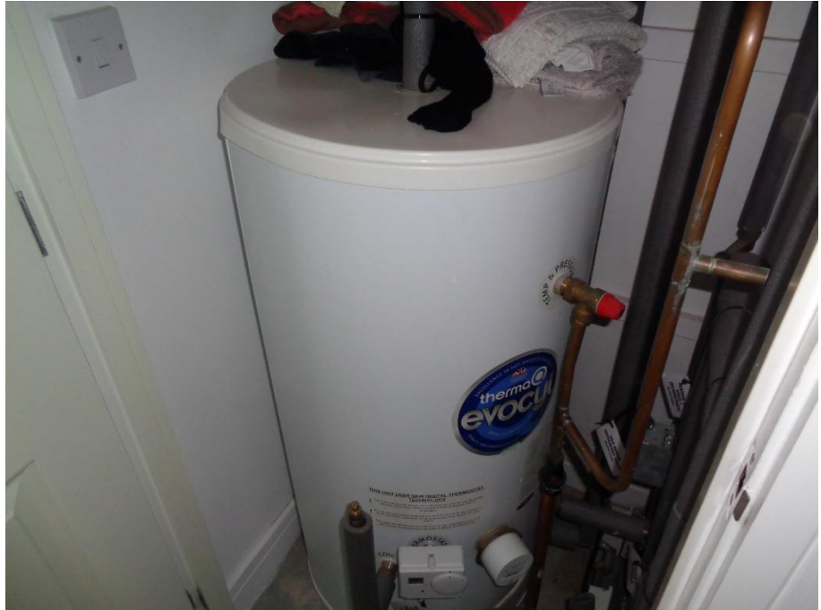
Pressurised hot water cylinder
