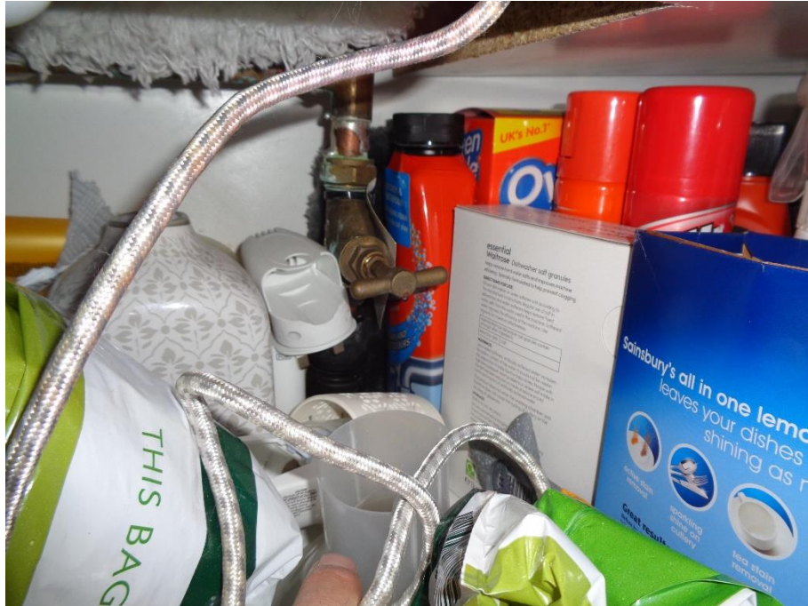
Stop tap under kitchen sink
