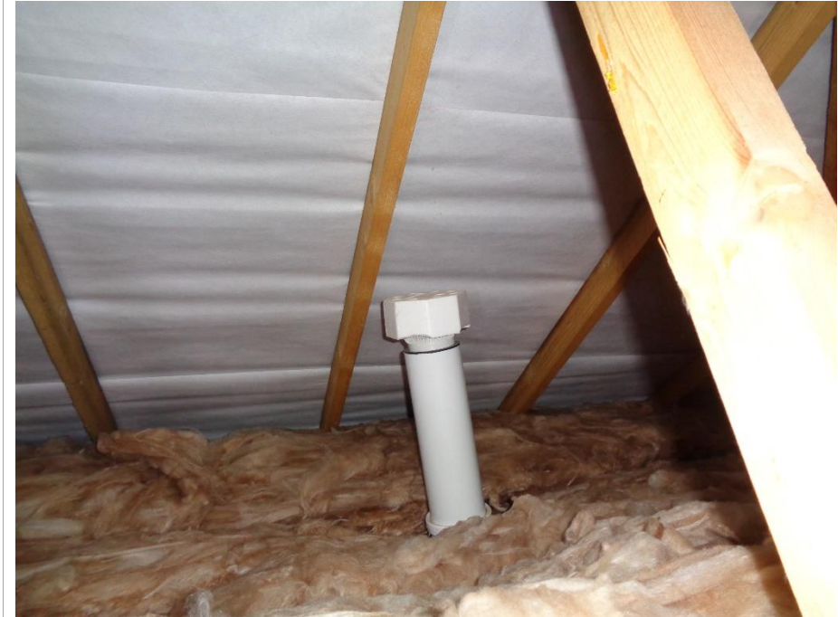
PVC soil vent with air admittance valve in roof space Condition Rating 2.
