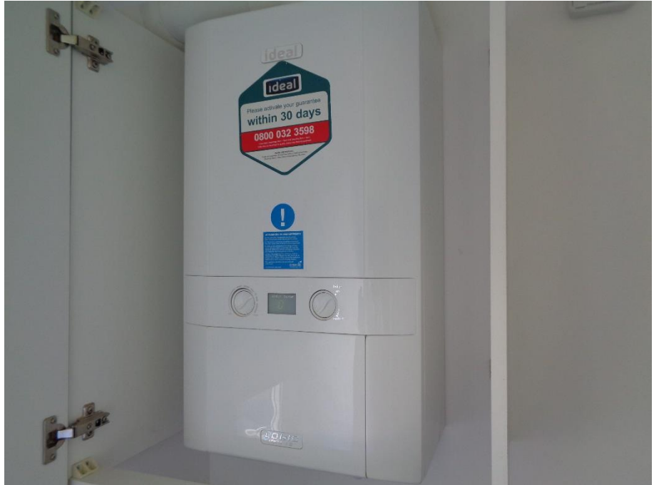
Gas fired boiler
