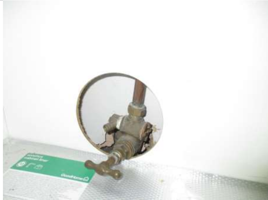
Main stop tap under kitchen sink
