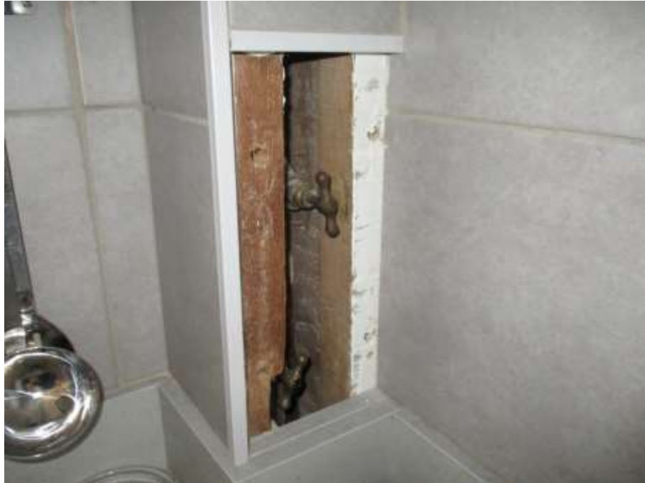
Additional stop taps in kitchen behind cover
