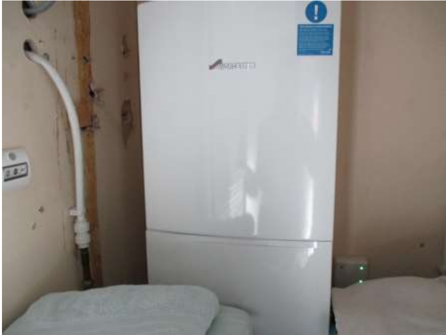
Gas fired boiler
